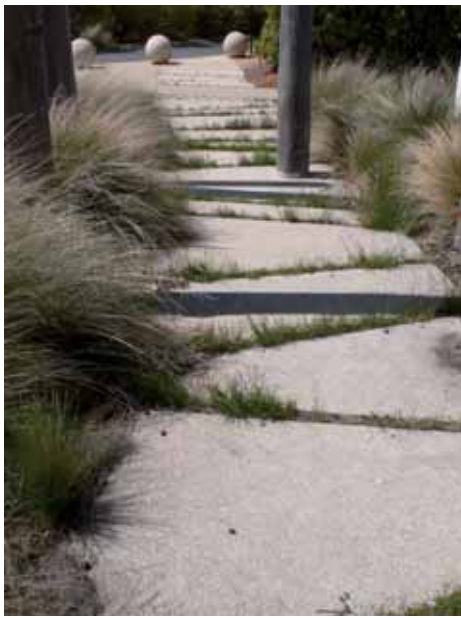
Wahlenbergia penetrate gaps between concrete path, ANU.
