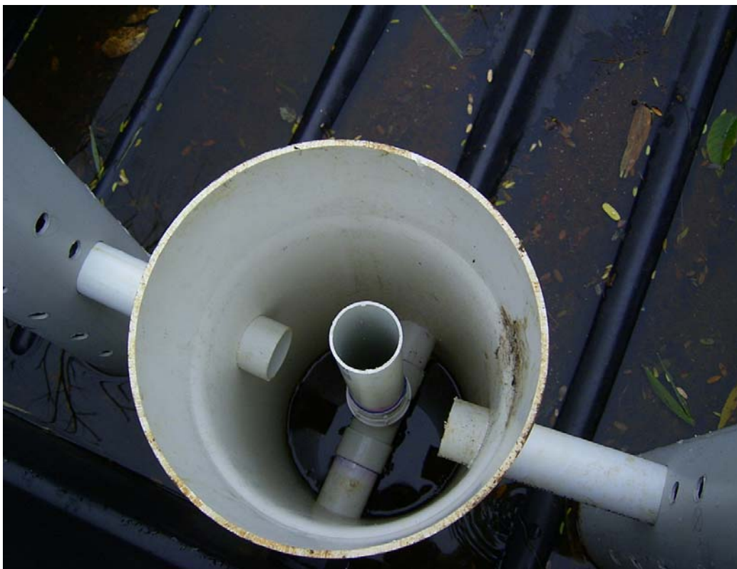
Water height adjuster inside a 300mm outlet tower
