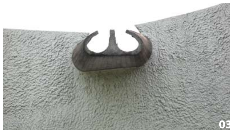
03 Off form finish to underside of concrete 'gargoyle' (for want of better descriptor) – just like internal ceilings by Robin Boyd at 218 Northbourne Avenue Canberra (AILA National Office)
